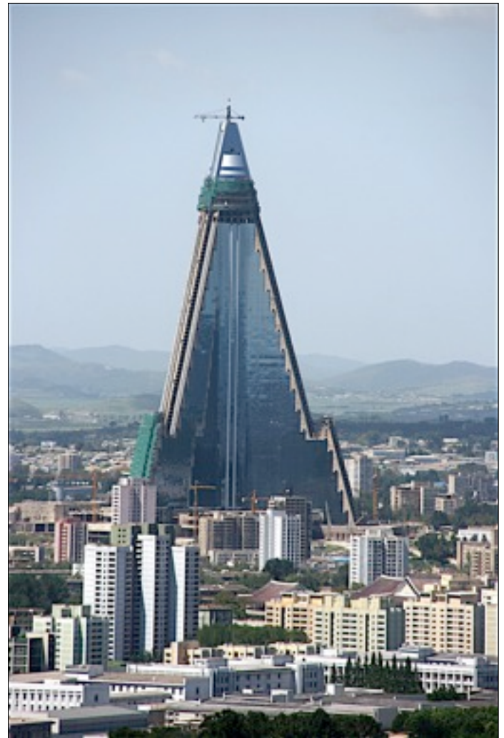
9.46 Construction of the Ryugyong Hotel began in 1987, and is due for completion in 2012 to mark the 100th birthday of Kim Il Sung.
